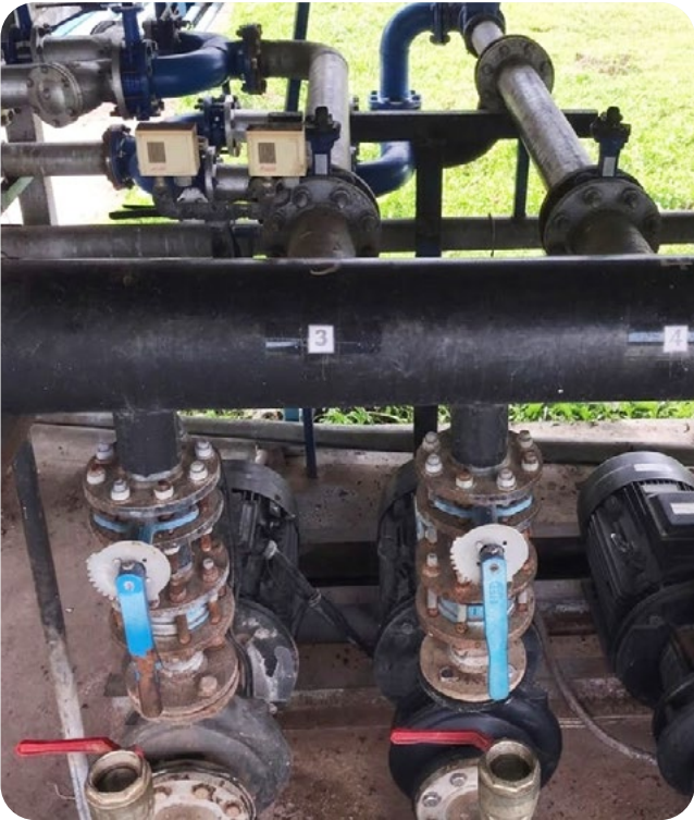
installation of additional water pumps, which allows us to double the water circulation rate from 350 m³/hr to 700 m³/hr
