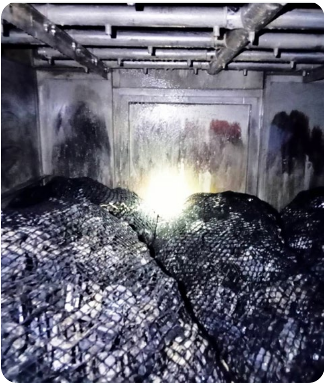
adding approximately 10,000 media units per machine to enhance pollutant absorption capabilities
